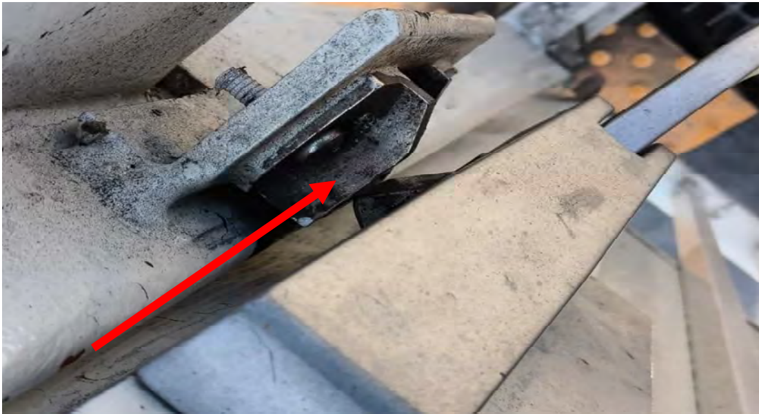
Leimert Park Station: 2024K-001 July 29, 2025 - Broken Latch
