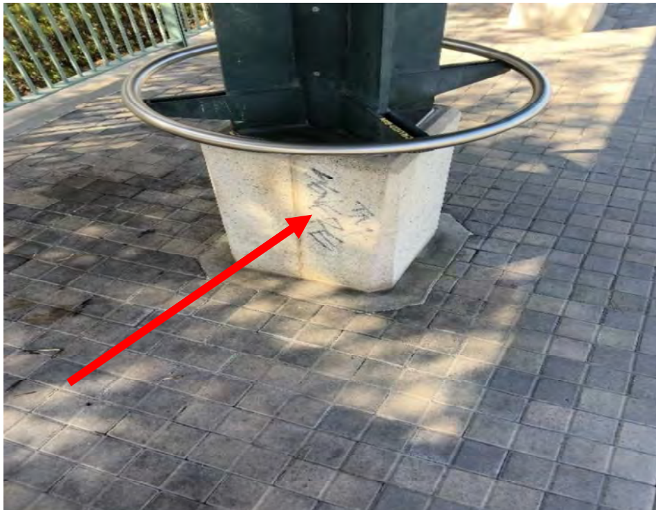
Lincoln/Cypress Station: 2024A-003 July 30, 2025 – Graffiti
