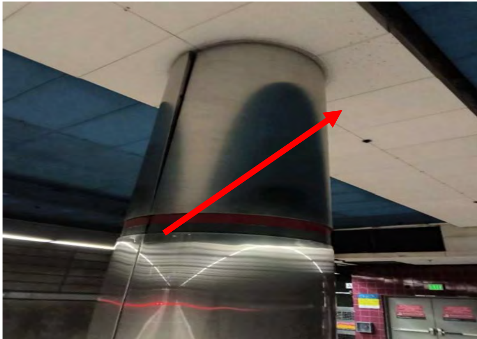
7 th Metro Center: 2024BD-001 July 31, 2025 - Detached Ceiling Panel
